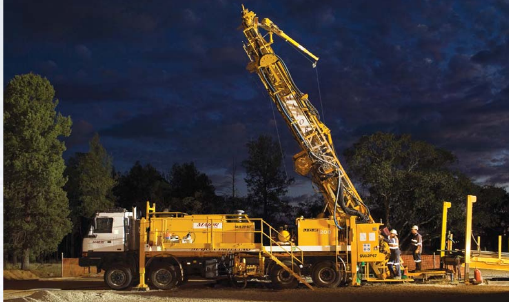
Above: UDR 1200 at work in New South Wales, Australia. Below right: Foreman and driller discuss safety procedures.
